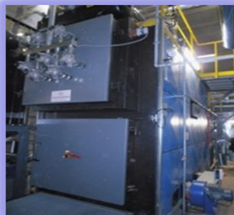
Mega Watt Biomass Boiler
