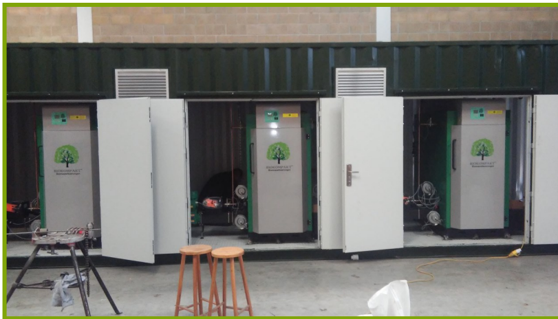
Three cascaded Biokompakt® boilers
