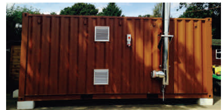
Biomass Boiler installed in 2014
