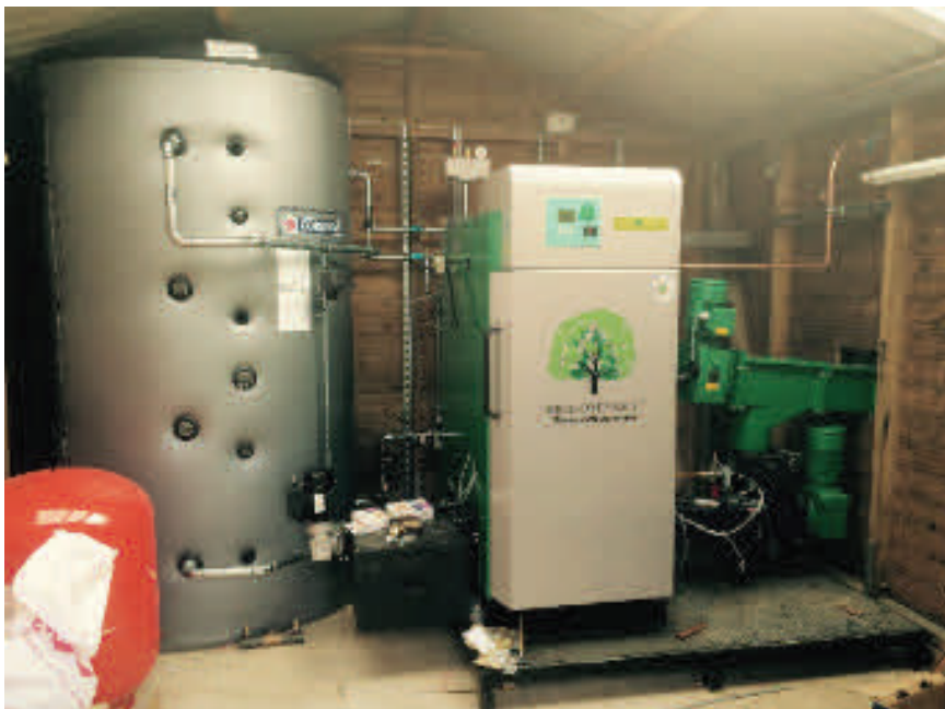
The Installation at Tiles Farm—Small Scale District Heat Scheme
